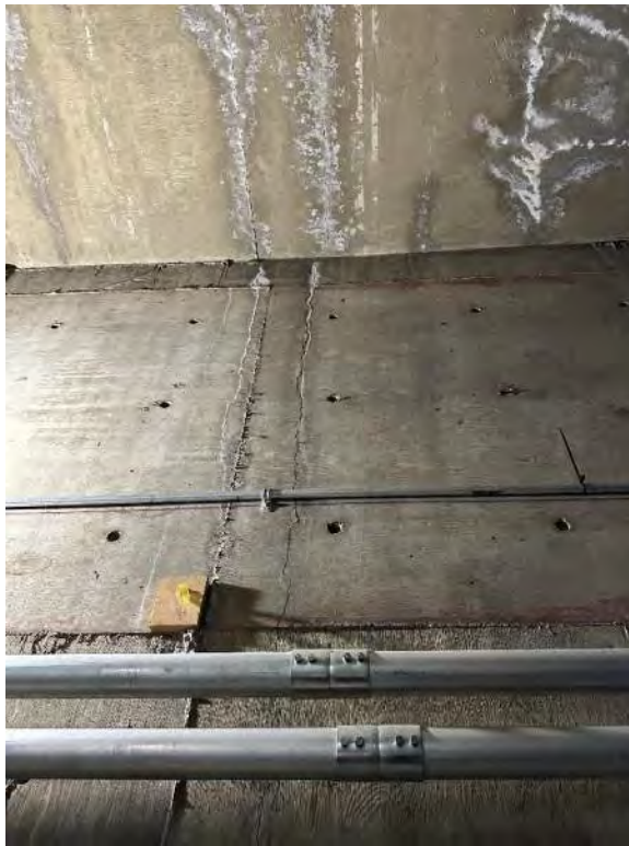
Photograph 8 – Cracking in concrete wall and efflorescence/cracking of slab in basement level
