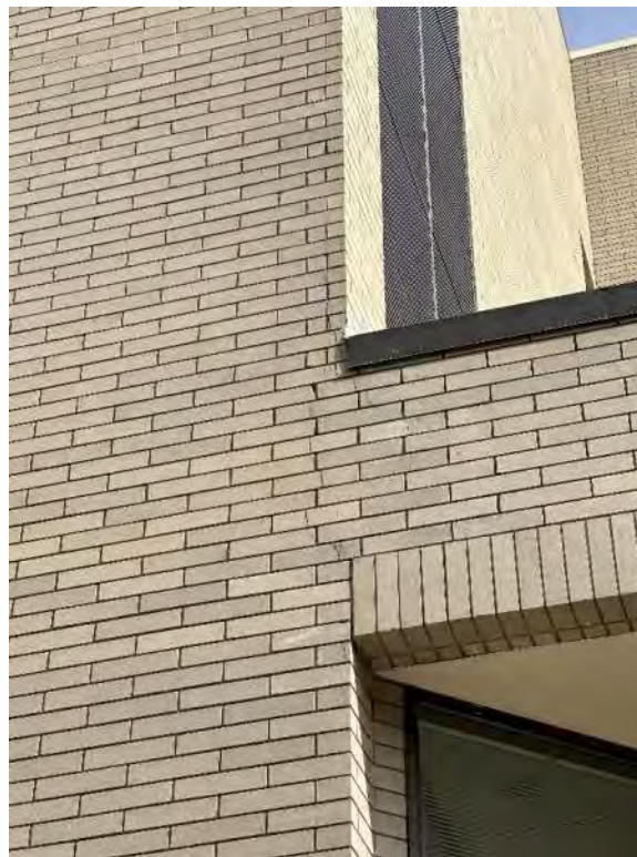
Photograph 14 – Cracking in exterior brick veneer
