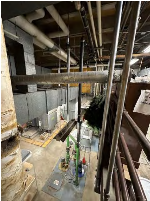
Photograph 2 – Laterally unbraced piping
