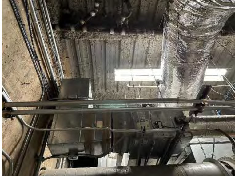
Photograph 5 – Laterally unbraced suspended equipment
