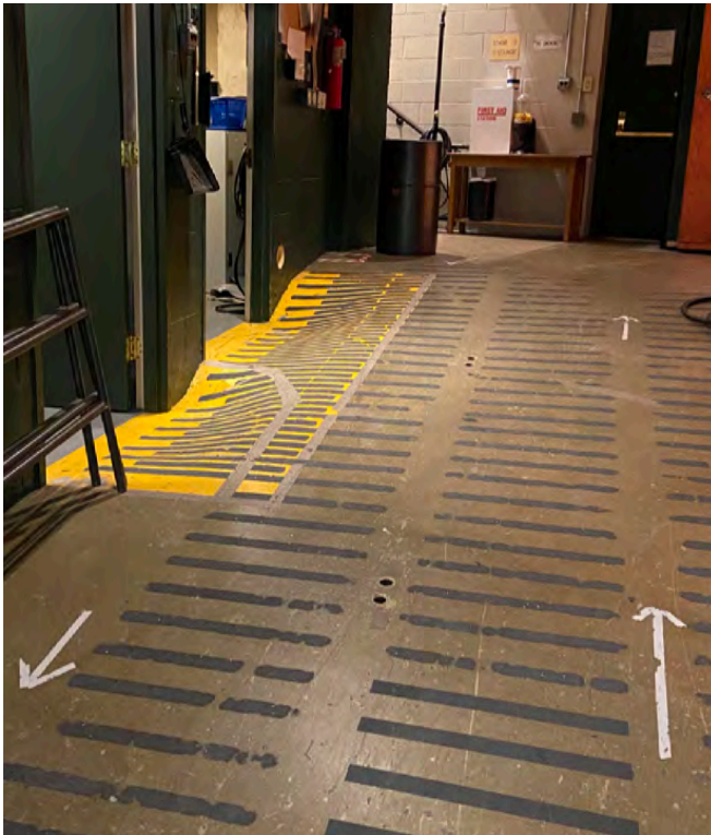
NON-CODE-COMPLIANT FLOOR SLOPES
