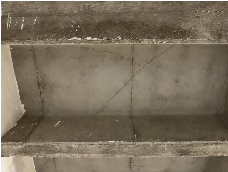
Photograph 9 – Cracking in concrete pan joists/slab in loading dock and storage area
