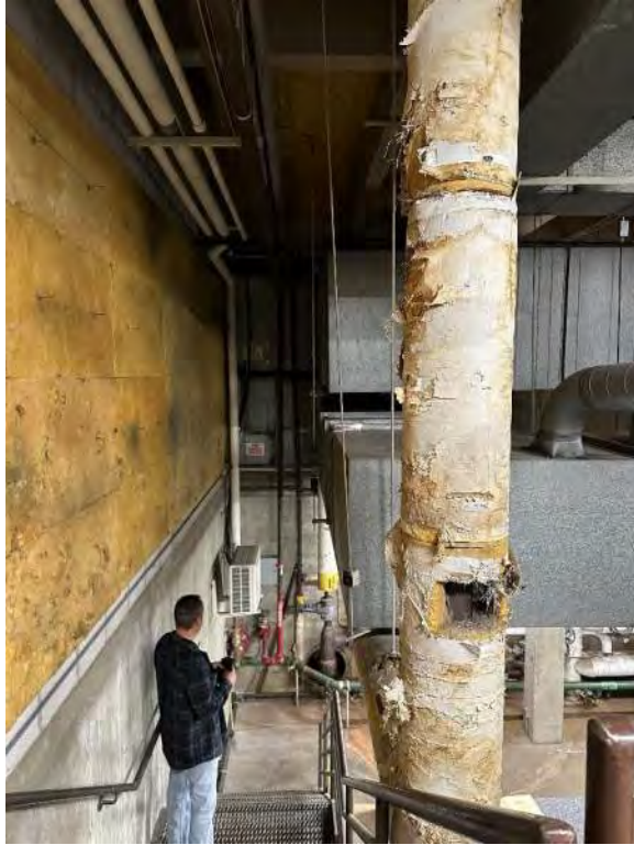
Photograph 1 – Laterally unbraced piping
