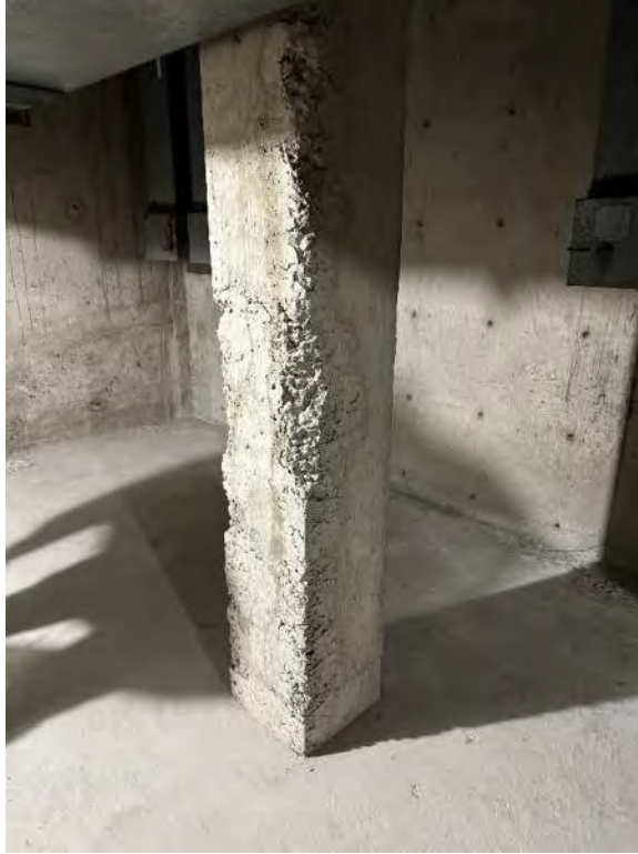
Photograph 7 – Poor consolidation of concrete column at basement level
