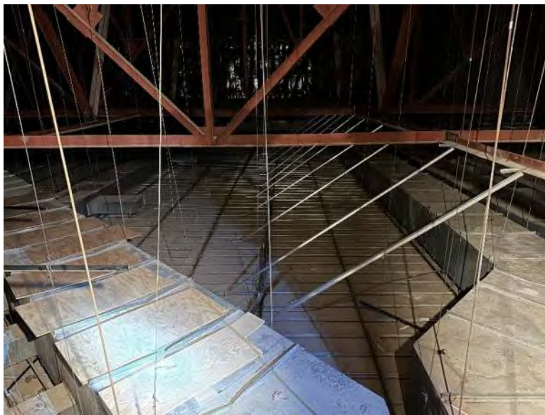
Photograph 12 – Bracing of suspended gypsum ceiling system
