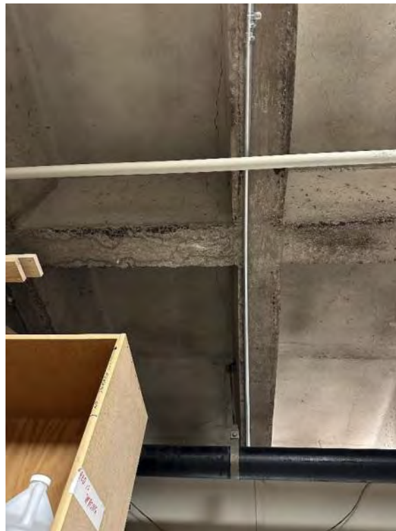
Photograph 10 – Cracking in concrete pan joists/slab in loading dock and storage area
