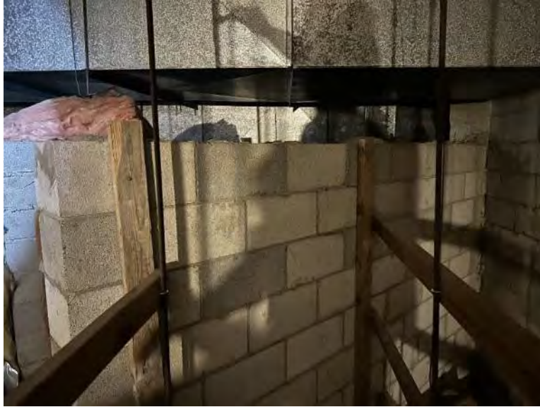
Photograph 13 – Laterally unbraced masonry walls at roof level
