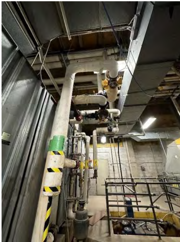
Photograph 4 – Laterally unbraced piping
