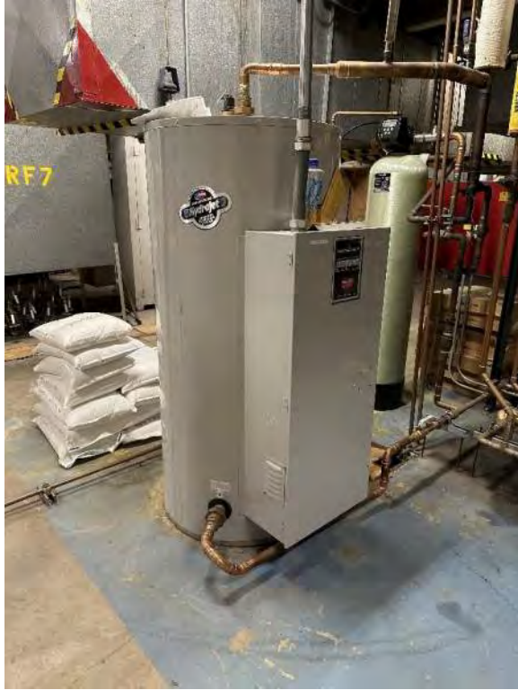
Photograph 3 – Laterally unbraced and unanchored equipment
